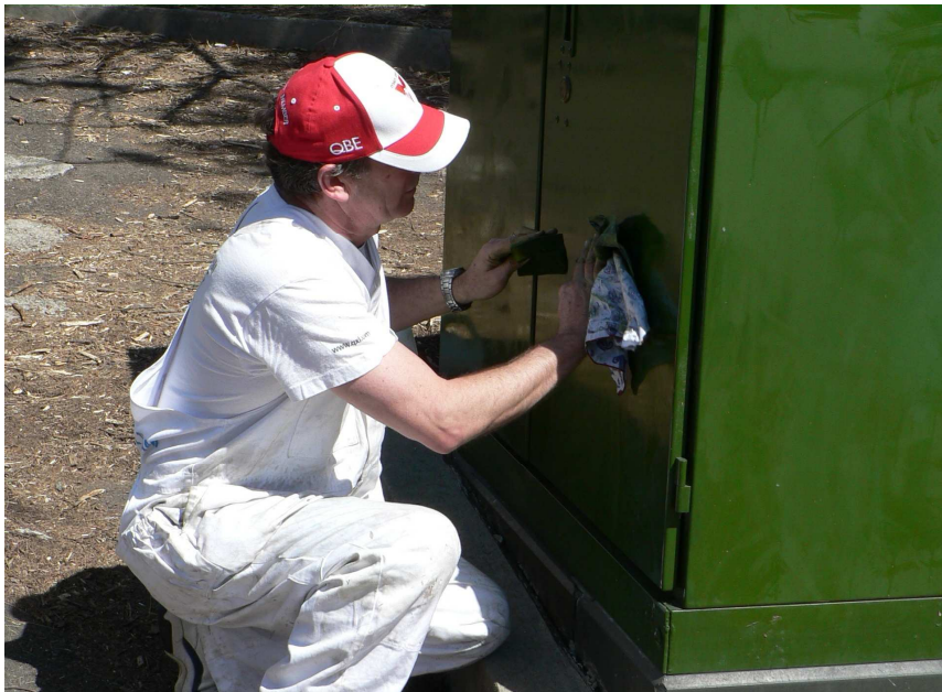
METAL SURFACES Rub off using graffiti solution
