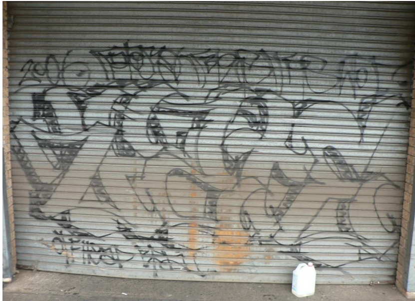
METAL SURFACES Rub off using graffiti solution
